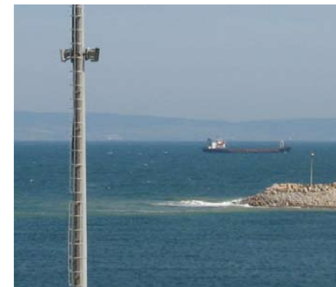
RSH-462 loudspeakers provide important safety announcements to incoming vessels at Icdas Jetty port in Turkey.
